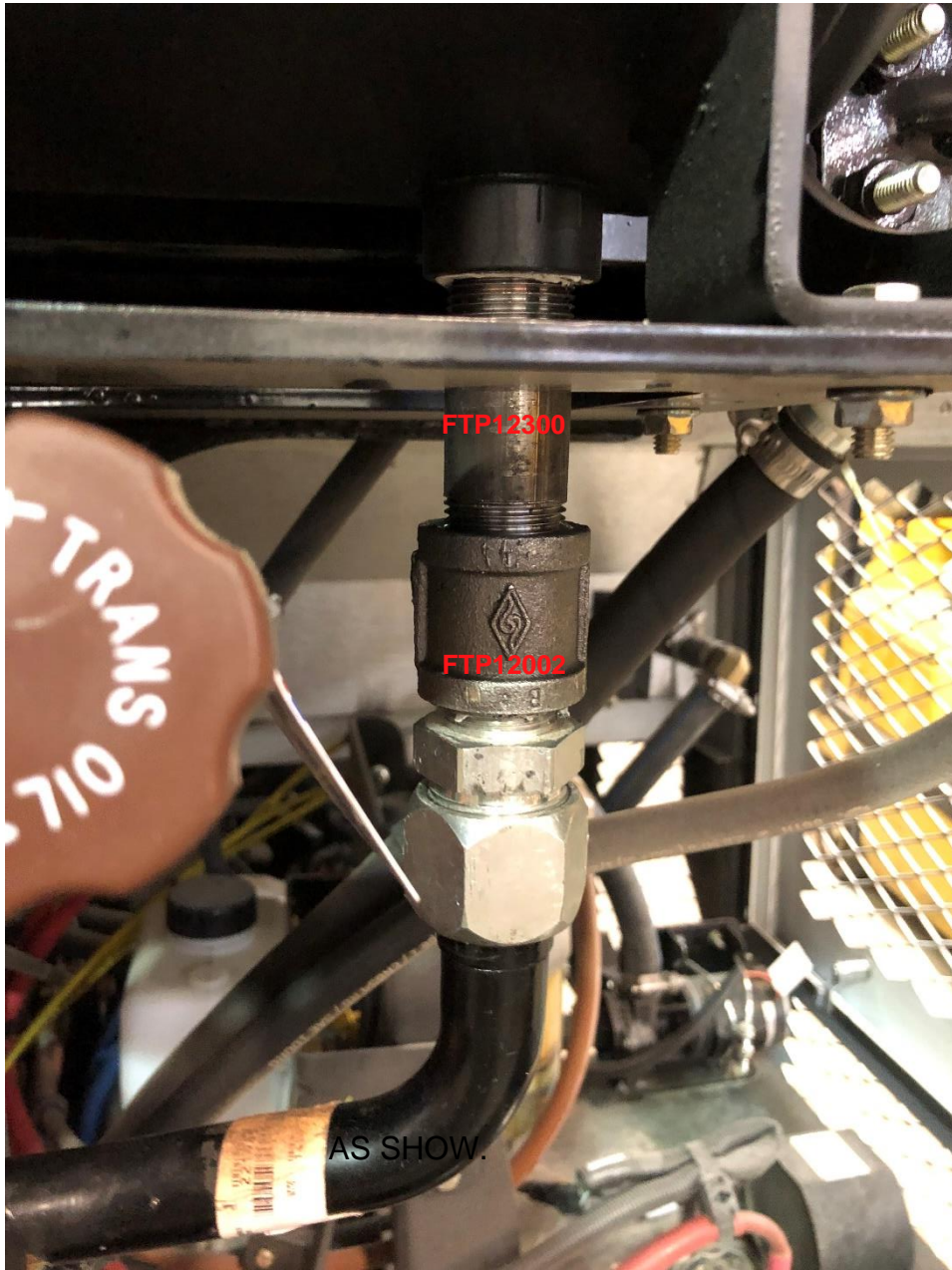
-DRAIN RESEVOIR TANK & ENGINE ENOUGH TO MODIFY THE OUTLET ASS'Y AS SHOWN.
