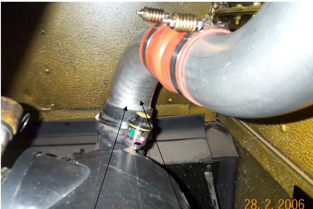
Note Air Filter rotation / This is the remant part of the cut part
