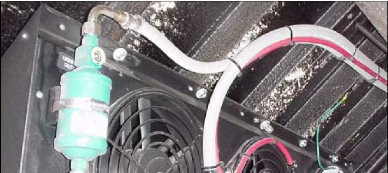
Figure 3-4 CM-3 Condenser Mounting (Typical)
