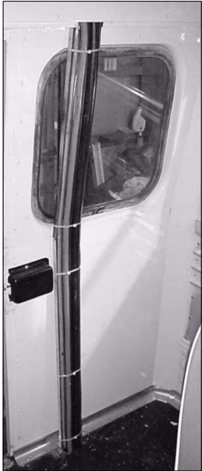
Figure 4-12 Hoses/Harness Secured With Tie-Wraps To Hose Cover Back
