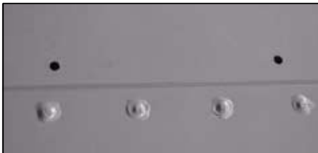
Figure 2-4 7/16 Inch Holes in Bus Roof
