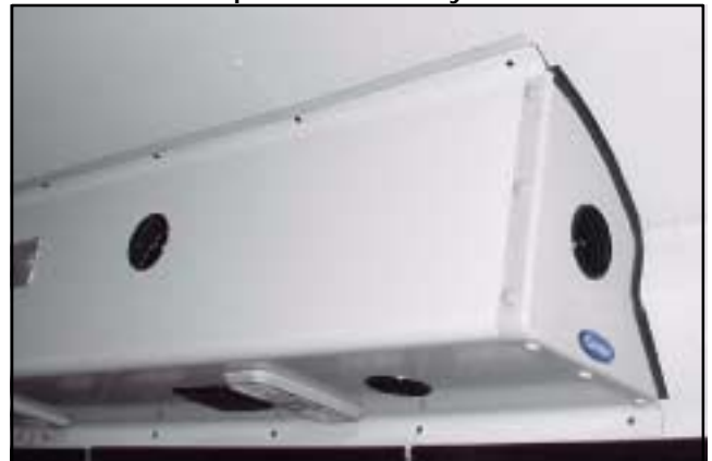
Figure 2-31 School Style Ducting-Drivers Side
